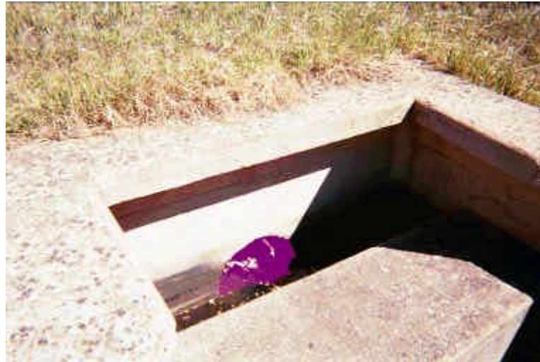
Outfall (highlighted in purple). Looking Northwest.
