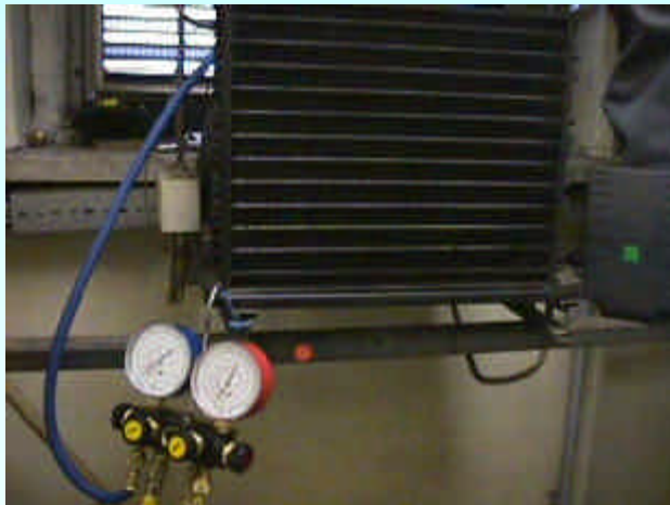
Refill unit w/new refrigerant
