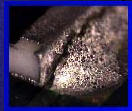
Cracked Solder Joint
