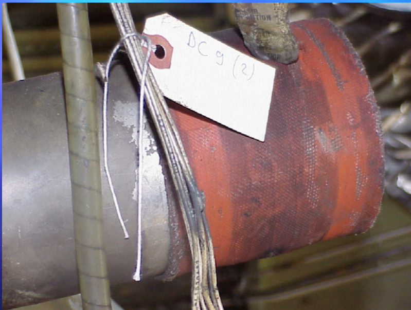
Contact with hot duct
