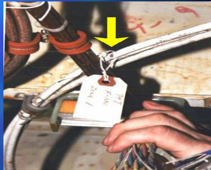
Power feeder chafing
