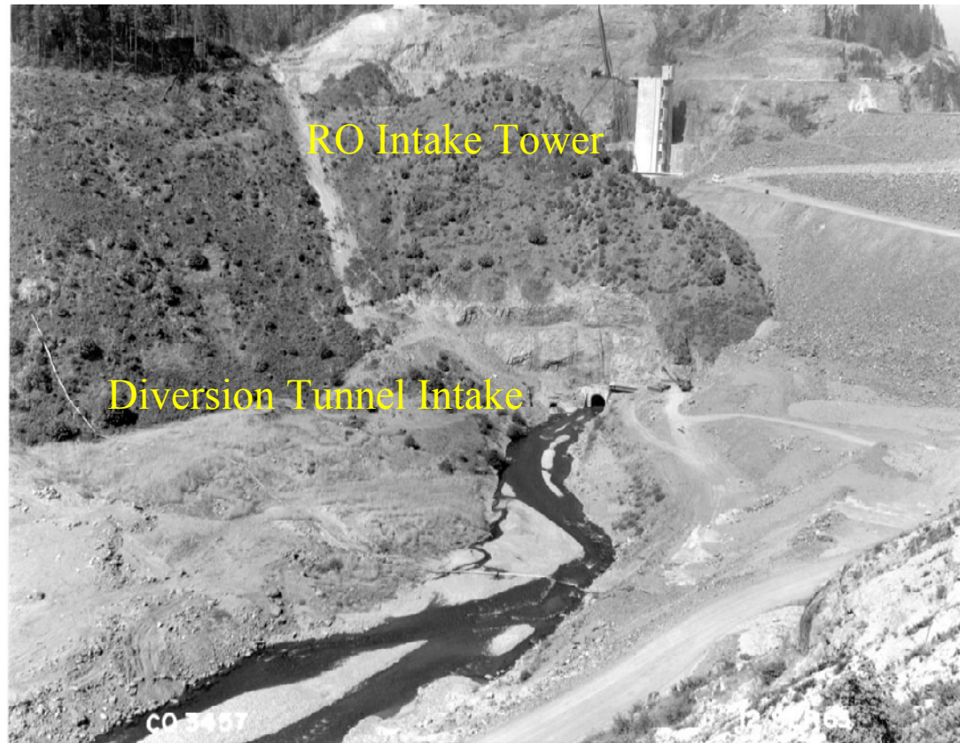
Construction photo, McKenzie River flowing into diversion, intake tower in background, Cougar Dam.
