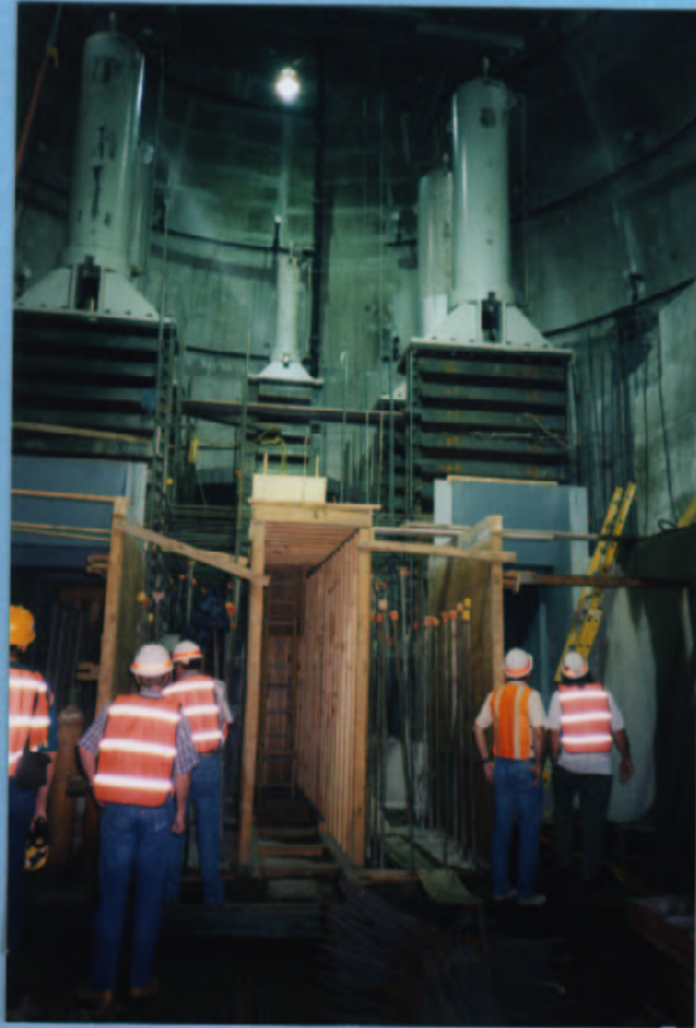
LOOKING U/S RO GATE FRAMES & ATTACHED BONNETS & CYLINDERS FORMWORK FOR GATE PASSAGES
