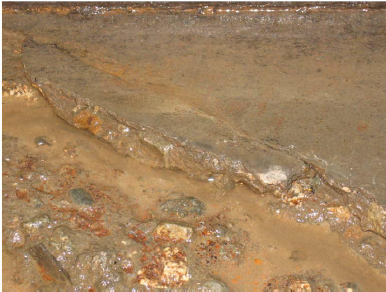
Fig. 3a – Cracking, delamination, and erosion of Slab 1 surface
