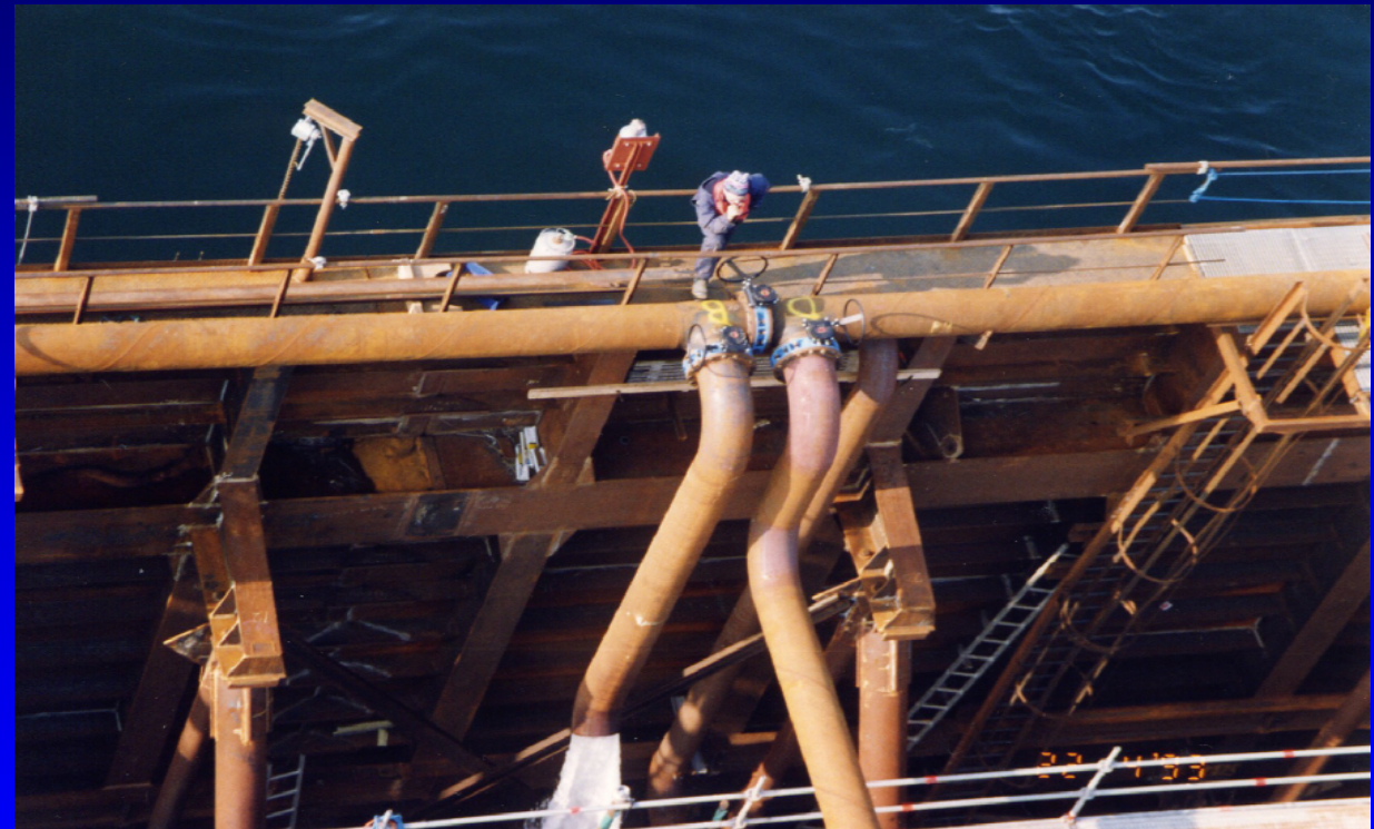
Piping Water Ballast System
