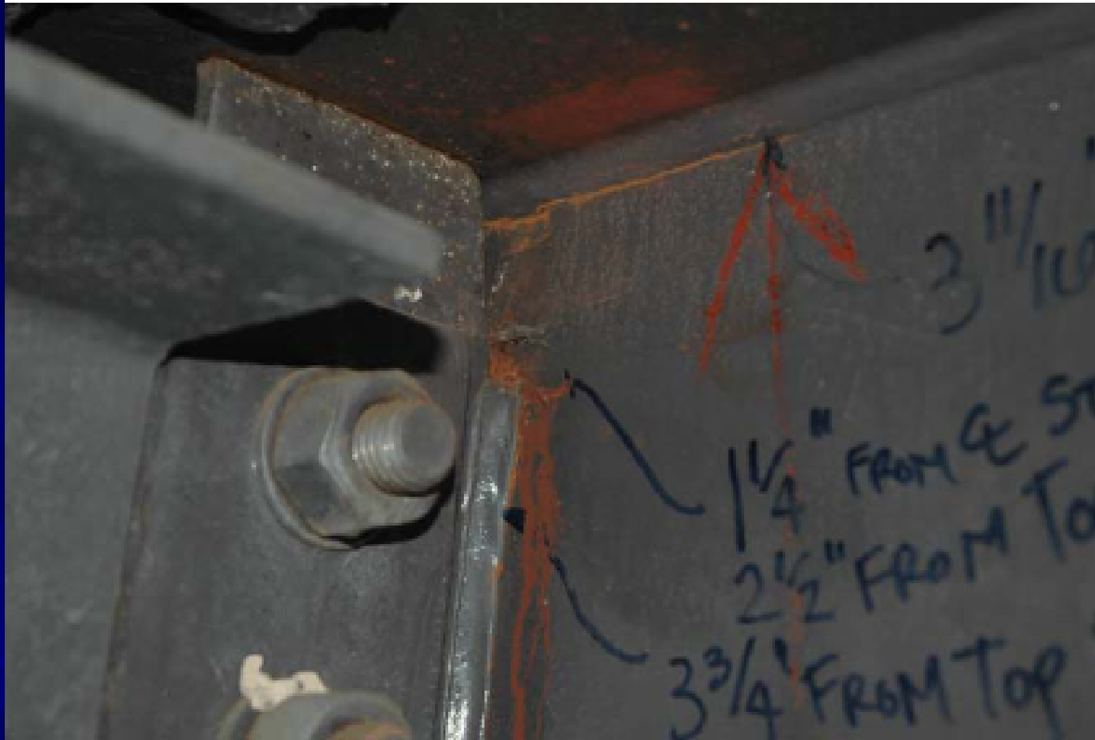
Web gap cracking at inside (upstream) face at Cross Frame 2, Span 4 of Girder A, Unit 2.
