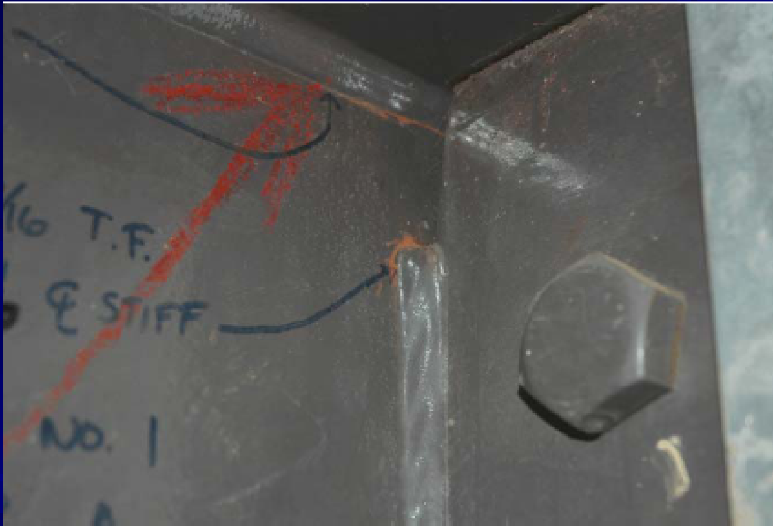
Web gap cracking at inside (upstream) web face at Cross Frame 1, Span 4 of Girder A, Unit 2.
