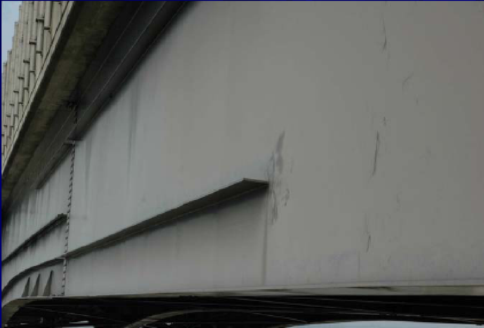
Longitudinal stiffener termination, Girder A', Span 11, Unit 3
