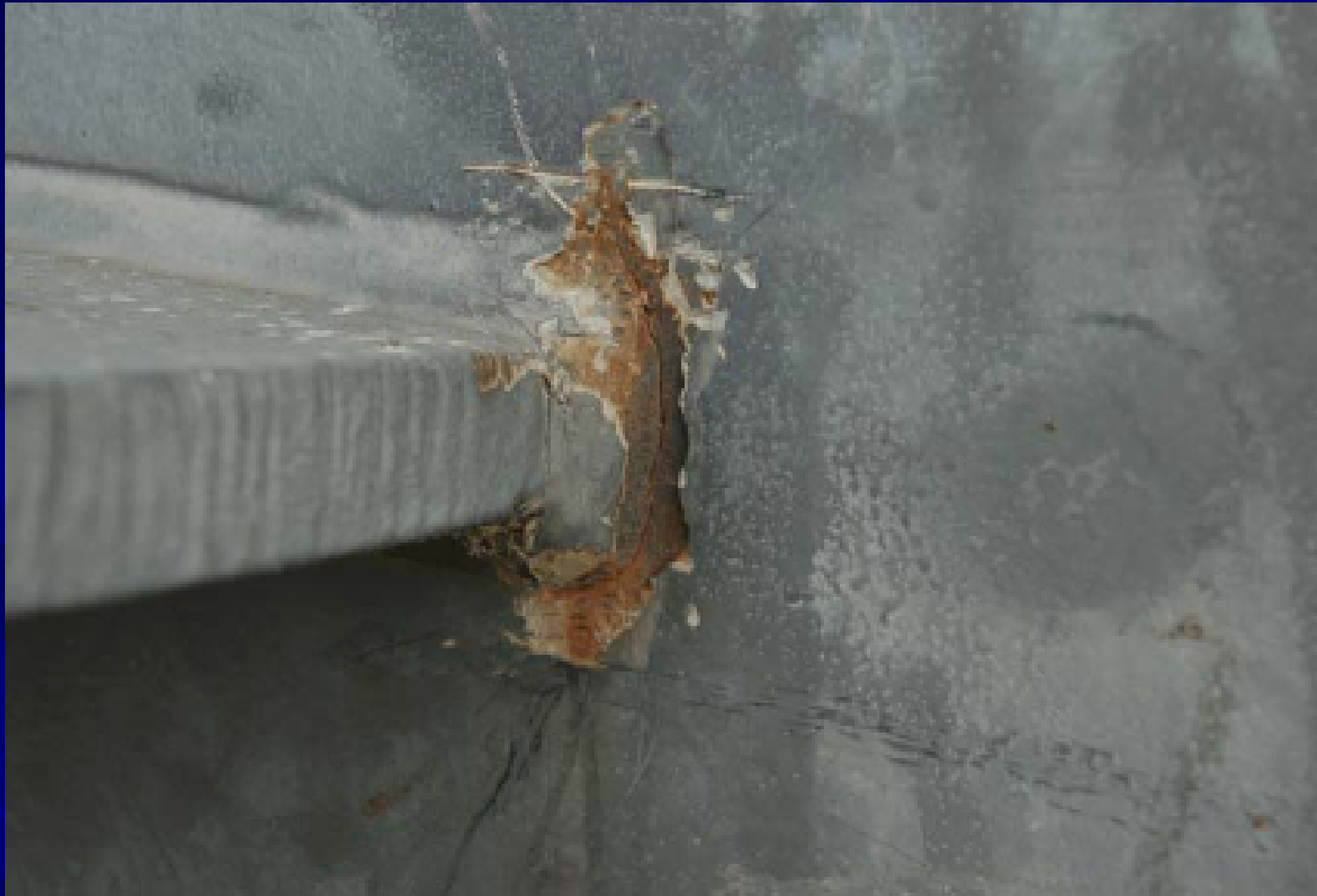
Close-up view of cracked longitudinal stiffener termination.
