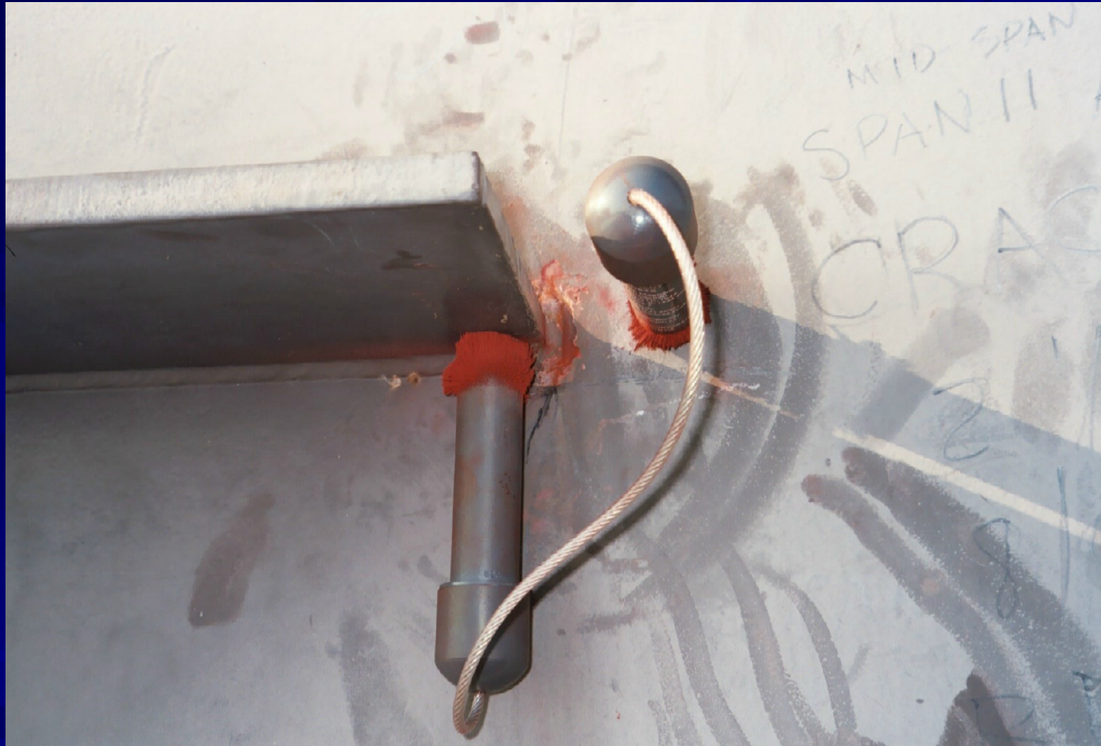
Crack at the Termination of the Longitudinal Web Stiffeners
