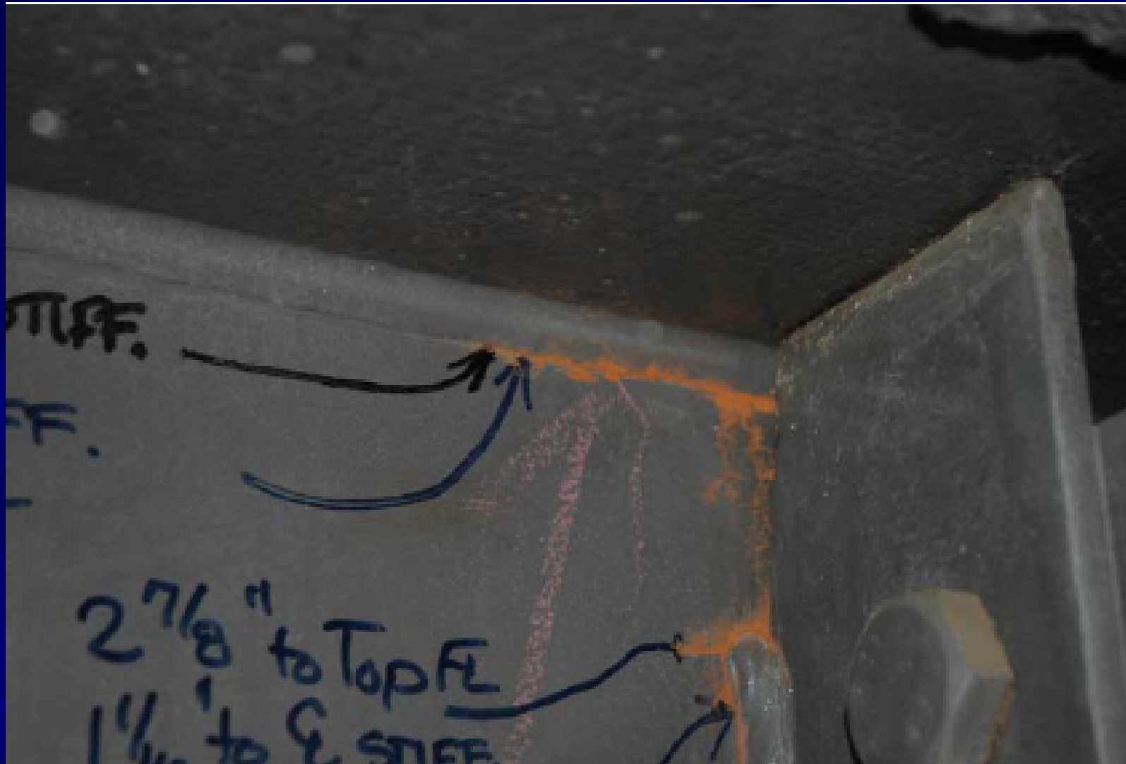
Web gap cracking at inside (upstream) face at Cross Frame 3, Span 4 of Girder A, Unit 2
