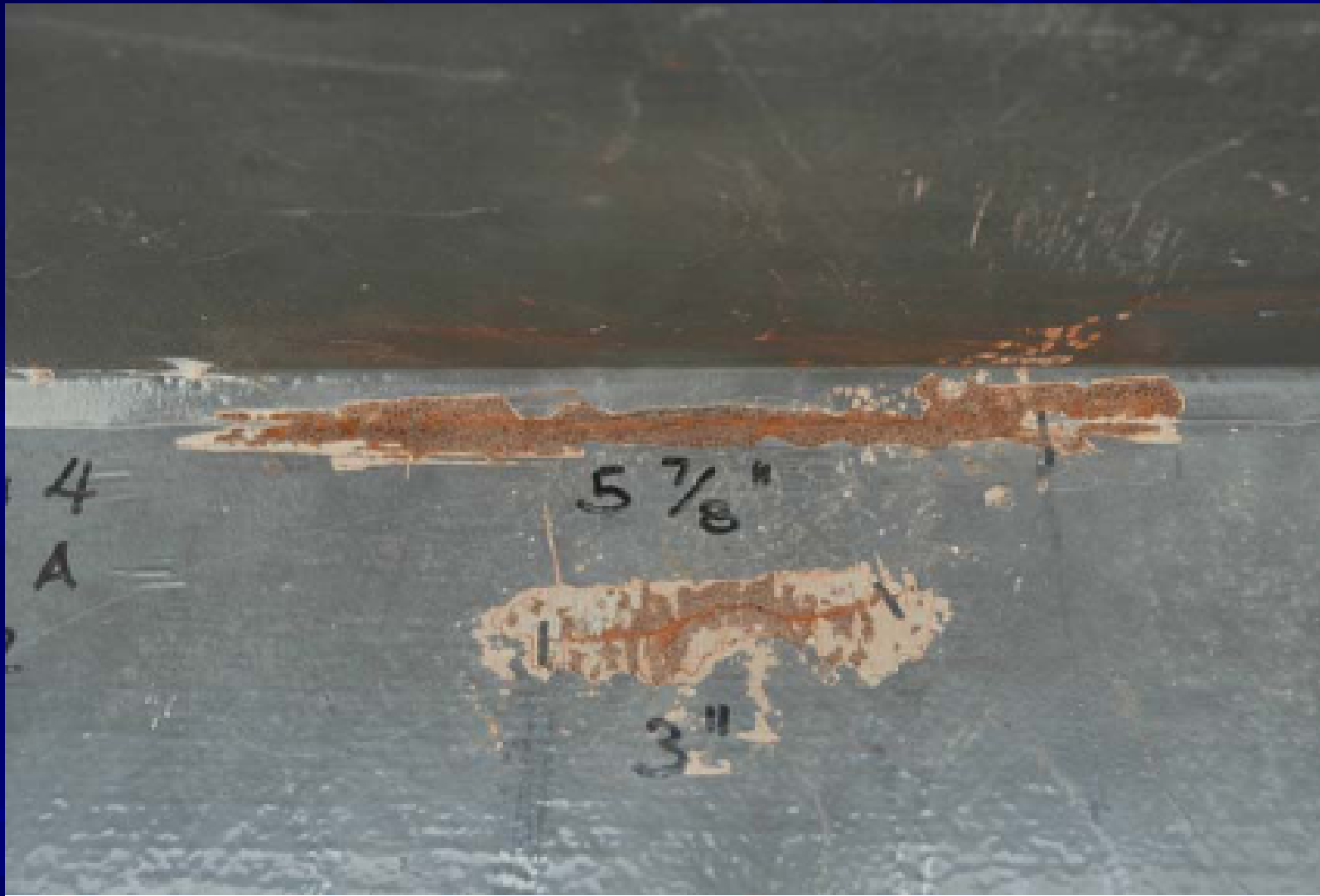
Web gap cracking at outside (downstream) web face at Cross Frame 2, Span 4 of Girder A, Unit 2.
