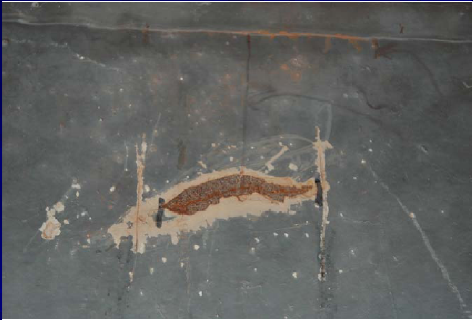
Web gap cracking at outside (downstream) web face at Cross Frame 3, Span 4 of Girder A, Unit 2.
