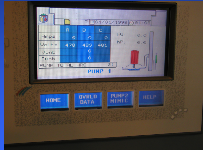
Pump & Sluice Gate Status Screen (MAGELIS Screen)
