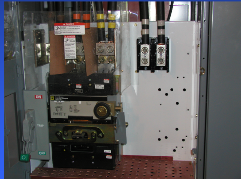
Dedicated Circuit Breaker for Generator
