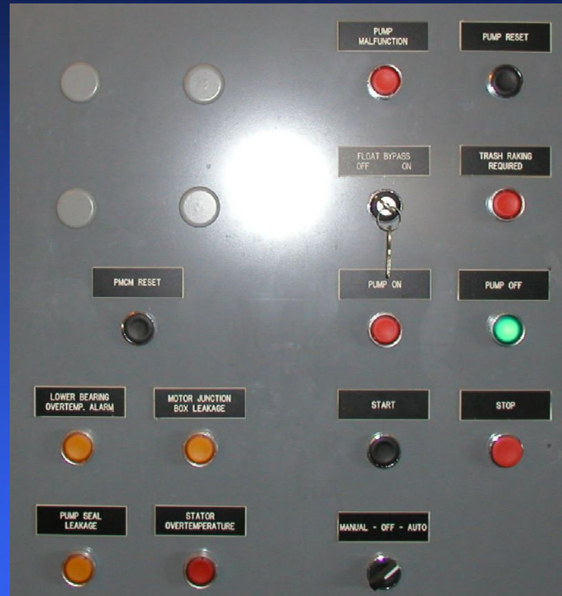
Pump Control Panel
