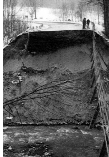
Chase Brook Bridge collapse caused by private dam failure, NY, 1996.
