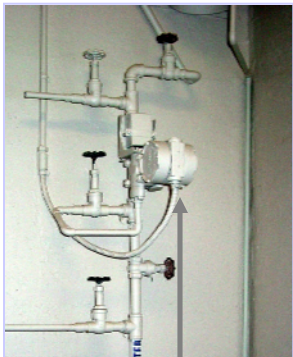
Tank 1 water level sensor at water plant
