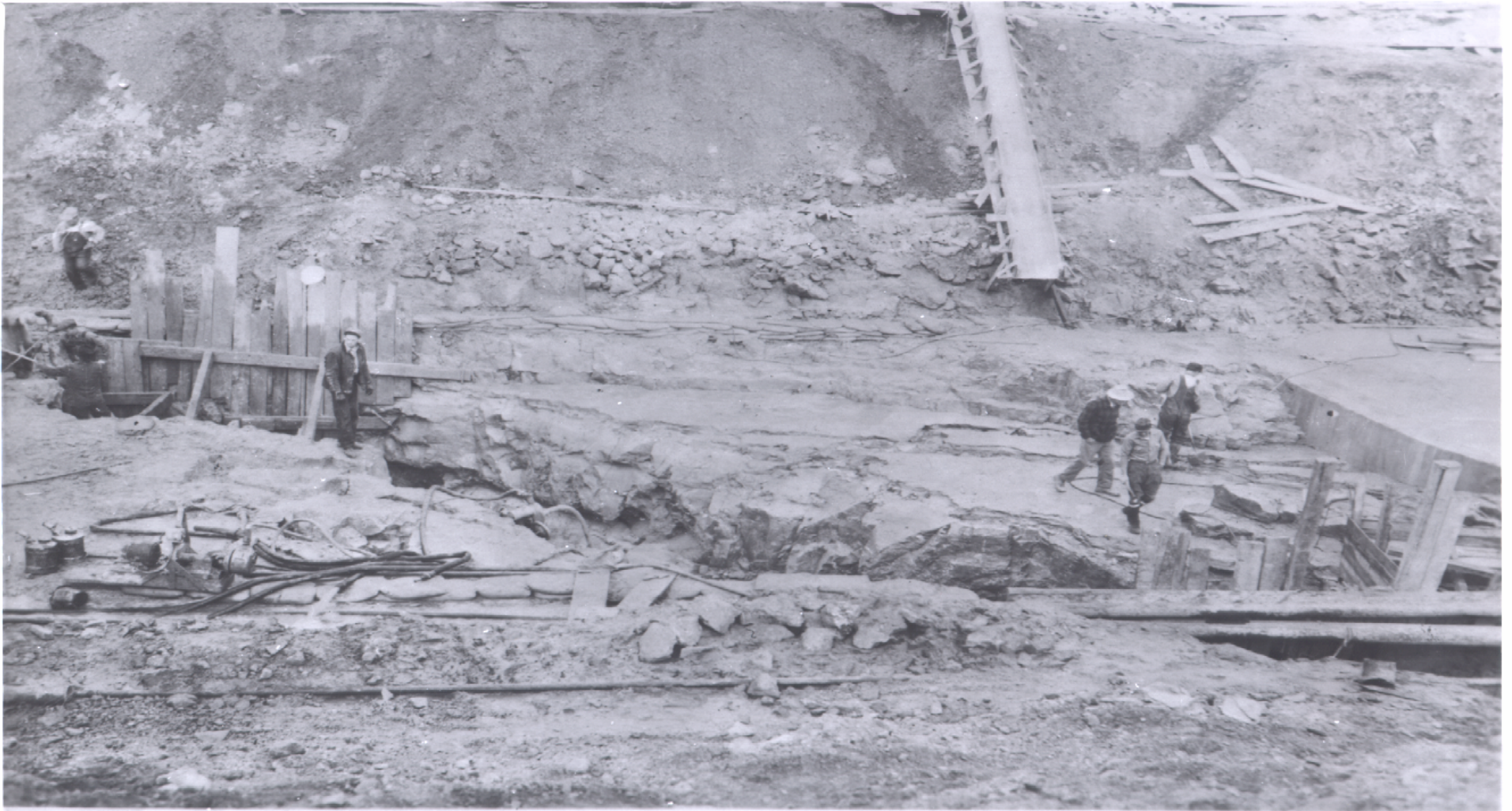
Looking NW from 35' U.S. of station 40 / 15: Open joint in cut-off trench foundation.
