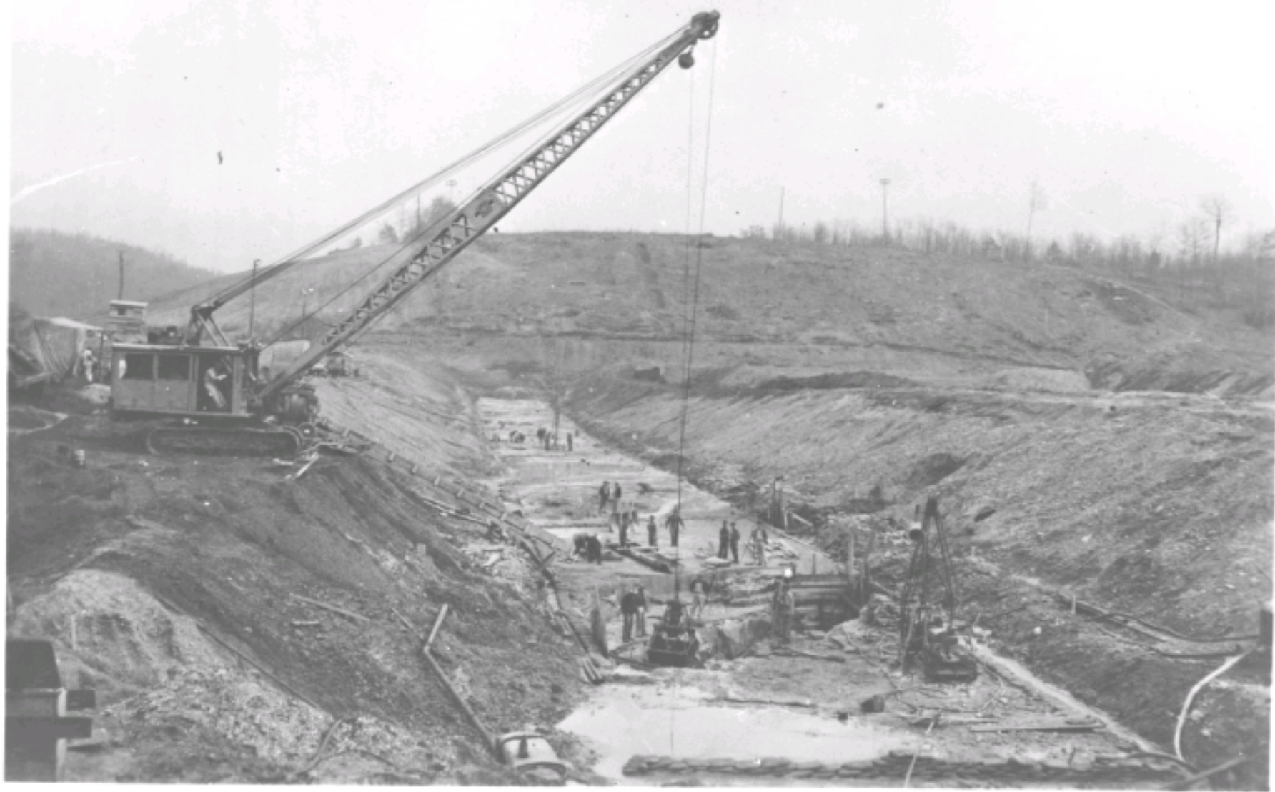
Looking E from 150' U.S. of station 41 / 68: General view of cut-off trench operations.
