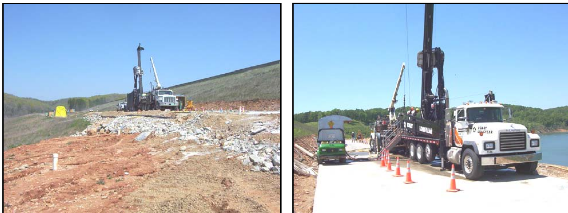
Figure 6. Long-stroke, truck-mounted rigs and tenders were used to pre-drill for the grout curtain at Clearwater Dam, MO (Boart Longyear Company, 2004)
