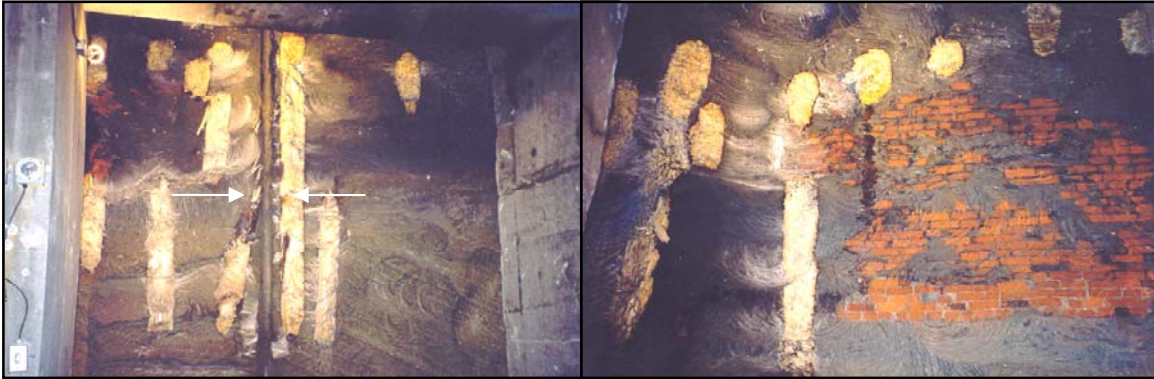
Figure 5. Penetration of Sonic drilling directly through wood piles, granite seawalls and brick foundations, Central Artery/Tunnel Project, Boston, MA (Boart Longyear, 1999)
