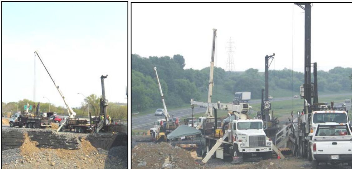
Figure 7. The use of Sonic methods to explore alternating Karstic voids to 450-ft below a bridge overpass foundation at PennDOT SR-33 (Boart Longyear Company, 2005)
