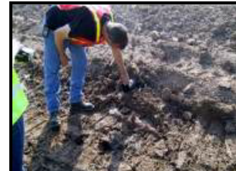
Proper drainage is required
