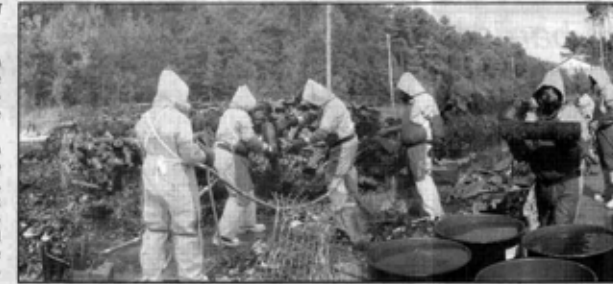
Workers with PIKA International clean what remains of a World War II-vintage warehouse that burned June 2005. The warehouse stored white phosphorus (WP) containers. Cleanup should be completed this month, according to the Directorate for Risk Management and Regulatory Affairs. (U.S. Army file photo)
