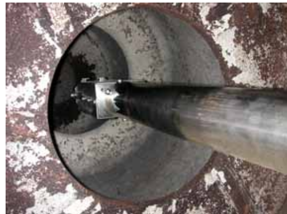
Debris discharge in RKS
