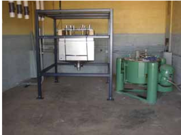
Sonication tank in bay 6A
