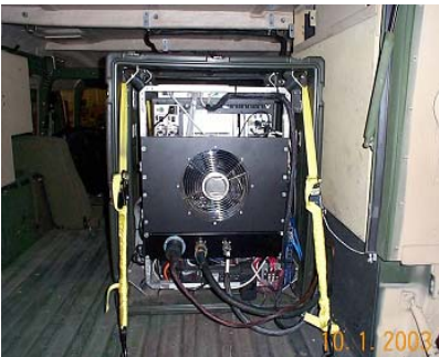
Before SprayCool: 482 Pounds & 17 Cubic feet
