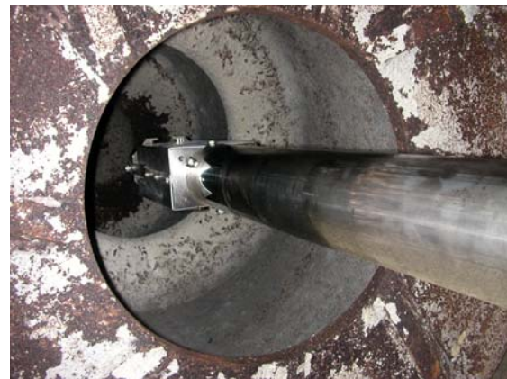
Debris discharge in RKS
