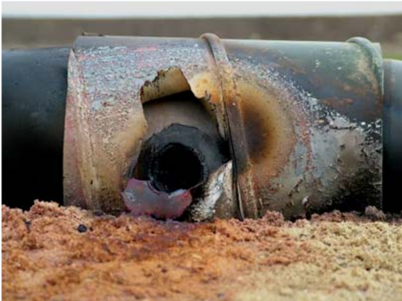
Impact hole – close up
