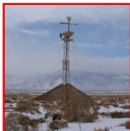
Remote Sensor Station
