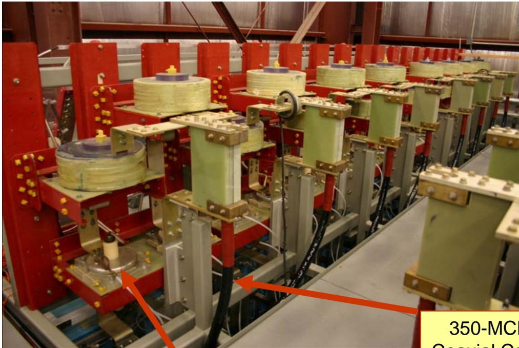
Spark Gap Switch
