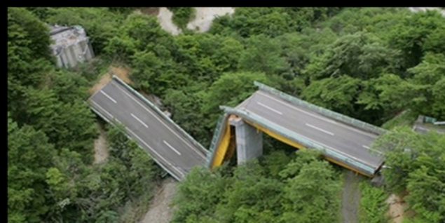
Earthquake – NE Japan
