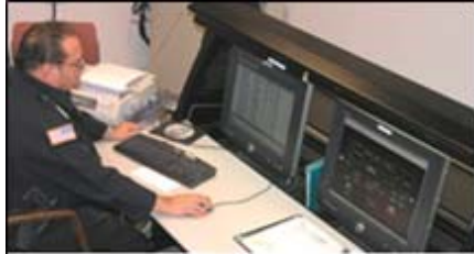
Integrated Commercial Intrusion Detection Systems (ICIDS)
