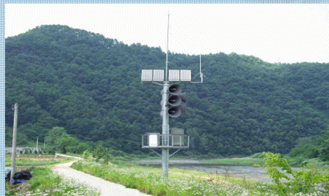
< Warn Alarming Station >
