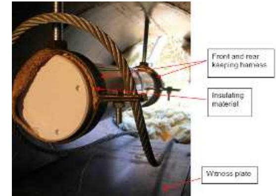
[ 21 ] SH PROTECTION CELL
