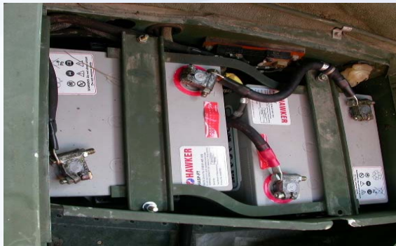
Current Lead-Acid Battery 24V, 65Ah, 120lb (2 batteries in series)
