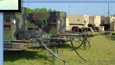
Central Power Solution
