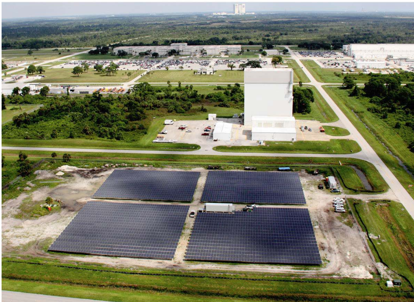
KSC 0.95 MW PV System
