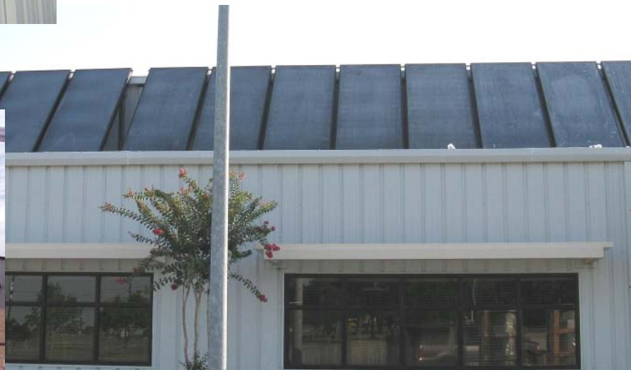
JSC Gilruth Center Solar Thermal Collectors
