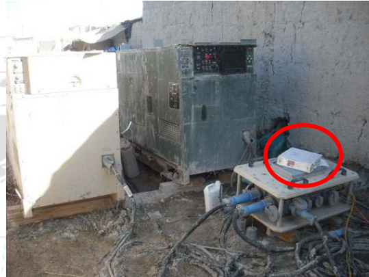
On the Job Training (Note: Generator Manual)
