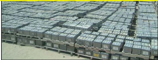
Bay of Batteries
