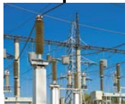
Utility Company Power
