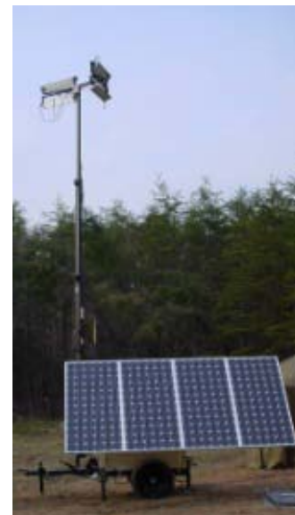
Solar Light Poles
