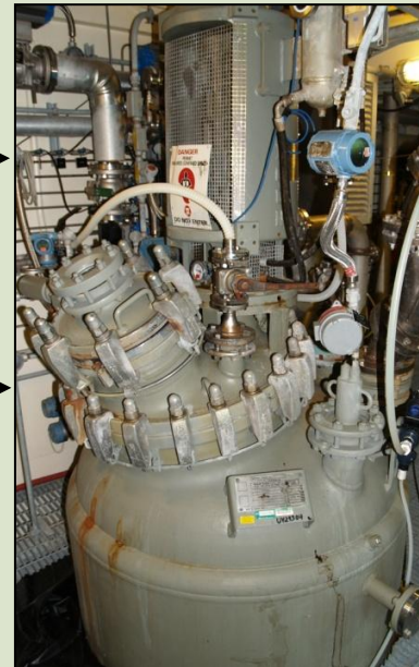
Jacketed, Glass-Lined Reactor System
