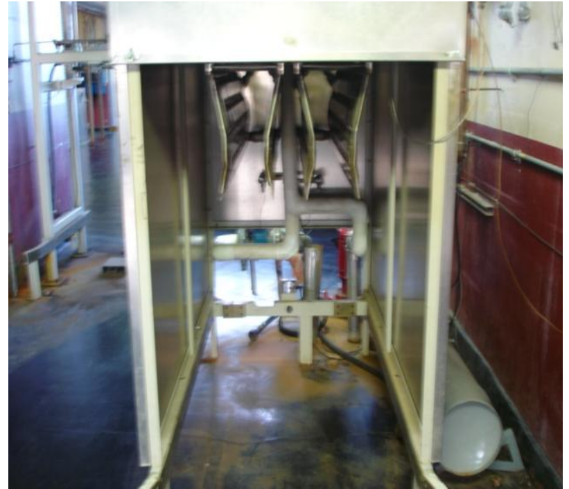
Water Cooling Oven
