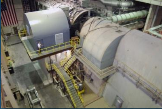
Compressor Research Facility
