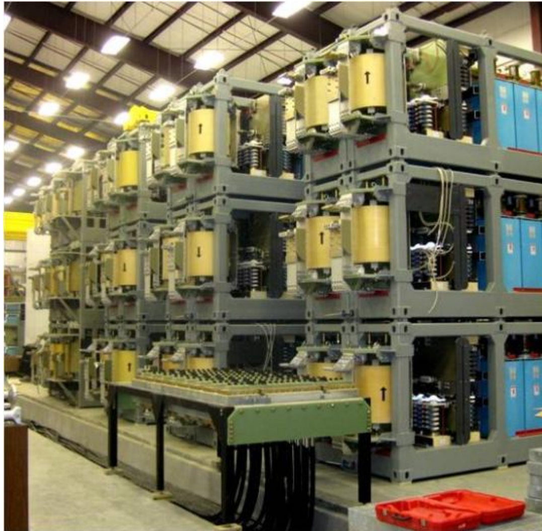
Pulsed Power at the Electromagnetic Launch Facility, Dahlgren, VA
