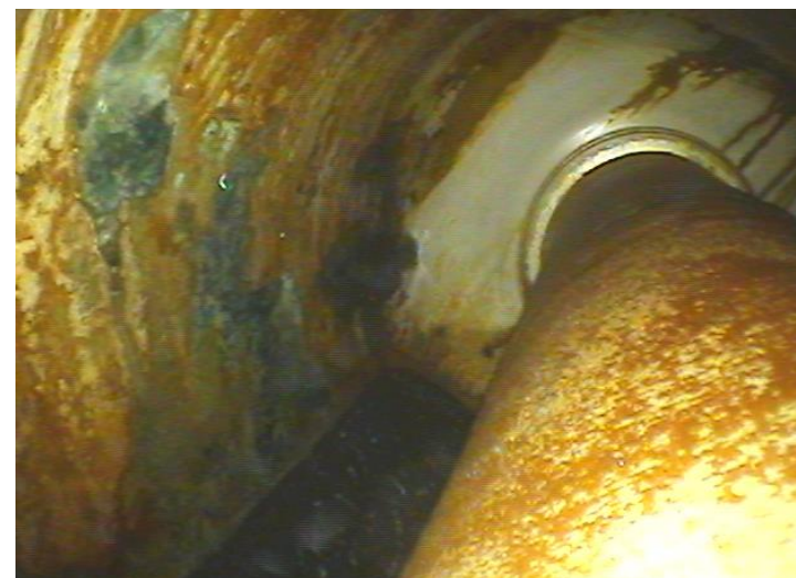
Solids in the IRFNA Tank
