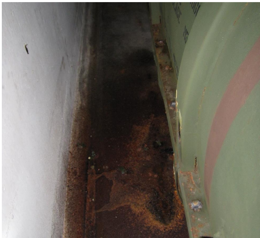
Nitric Acid Accumulation on ECM Floor
