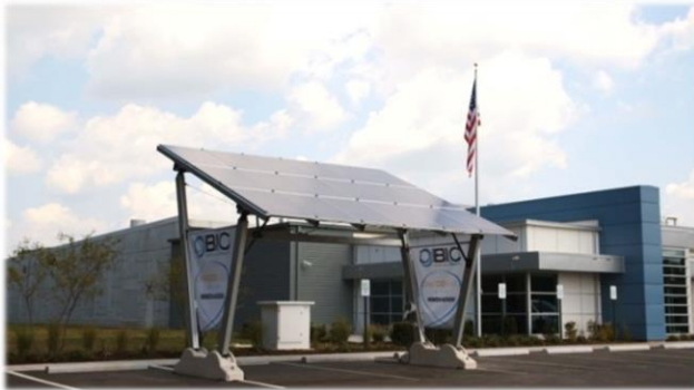
Solar Array with Integrated EV Charging
