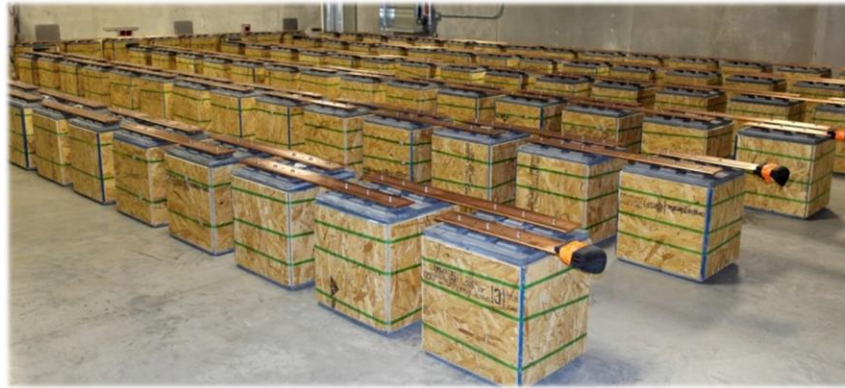
Large Grid Storage Device (approx. 1MW)
