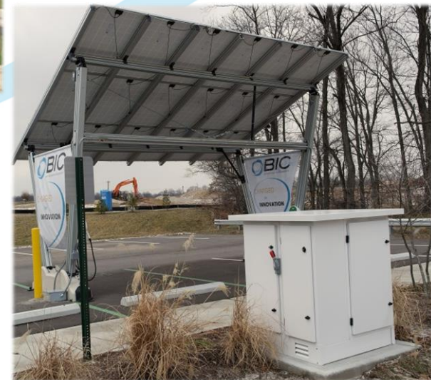
Integrated Power System (IPS) Supporting Solar and Wind Data Collection and Remote Management
