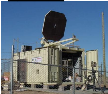
AC Wall Power Stationary
