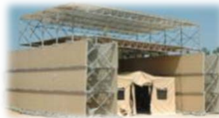
MPS w/ Overhead Cover for Critical Assets
