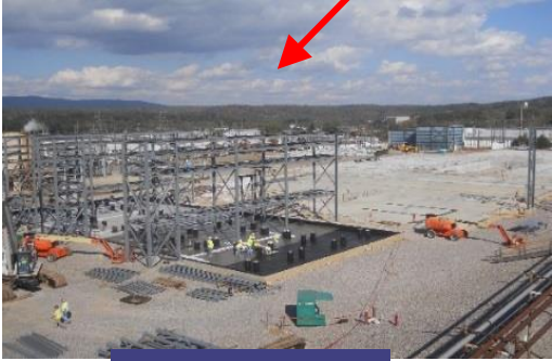
Acid Tank Farm
