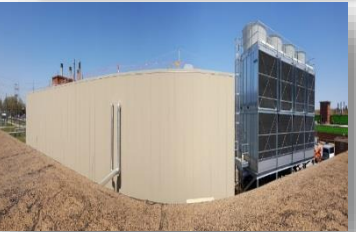
Lake City AAP HVAC New Central Utility Plant (CUP)
