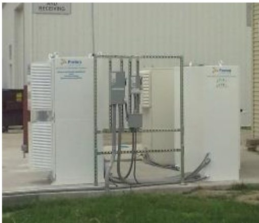
Silent Camp energy storage system installed at ERDC/CERL test site
