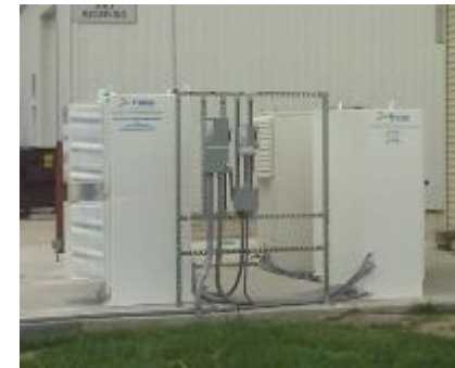
FOB Energy Storage
