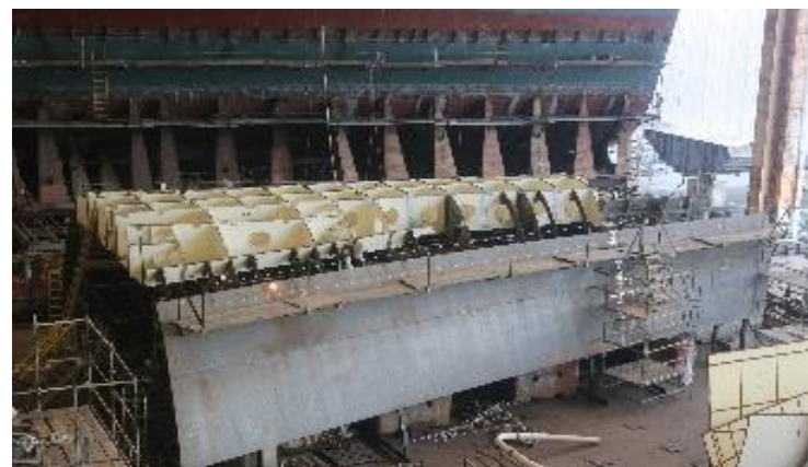
Ballast Tank and VCHT Room #1
