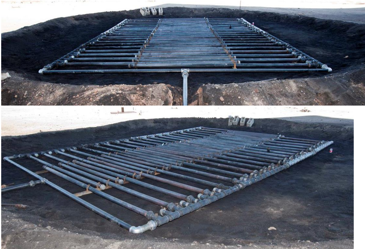
Figure 2. Modified 4.6 m by 6.1 m Burner
