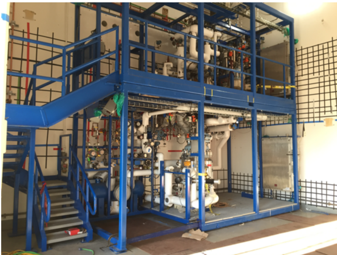
Figure 4 Pilot skid installed at LLNL Site 300.
