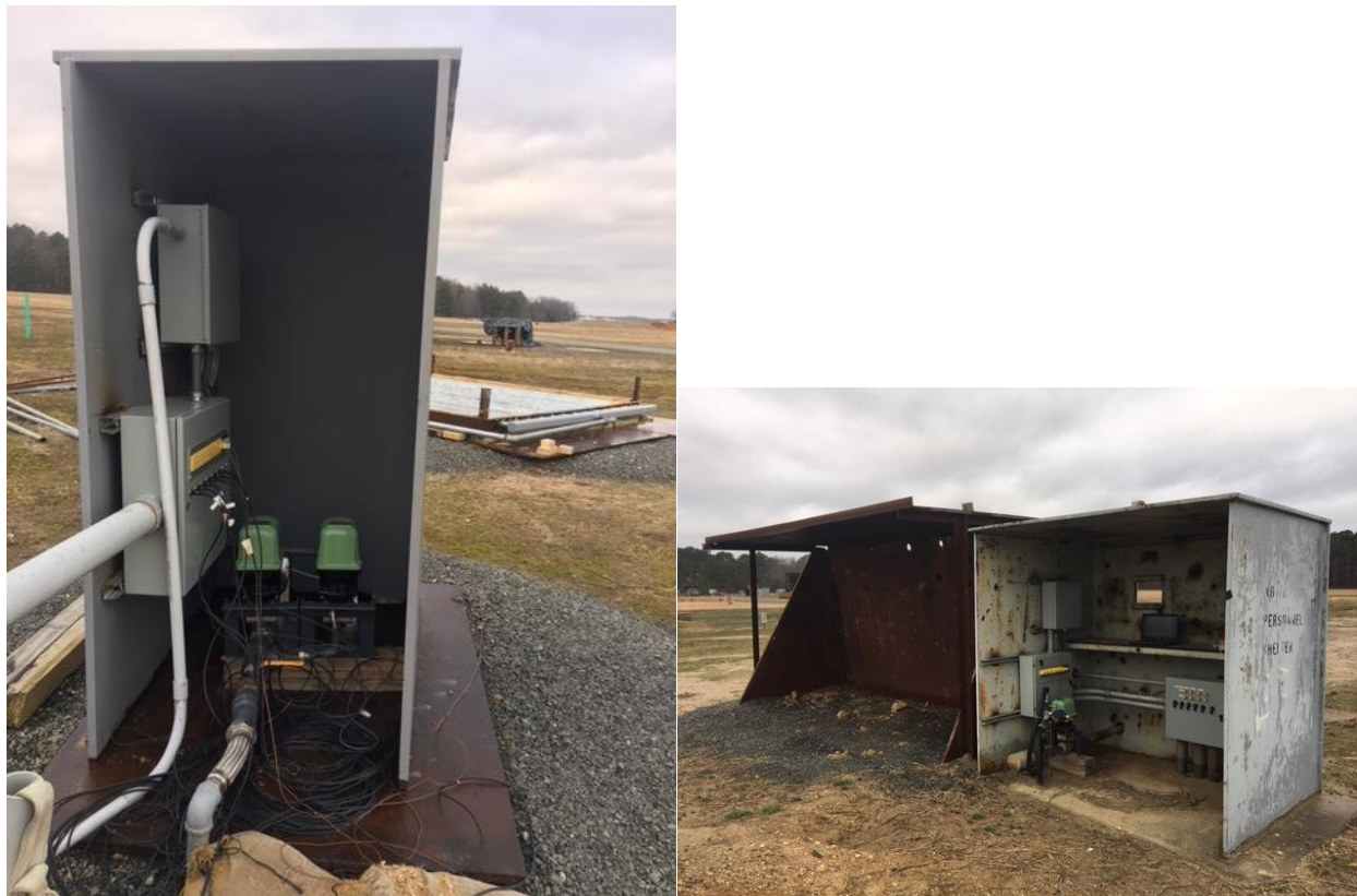
Figure 5. Shelter for the fuel delivery and pressure regulation system equipment and shelters for propane tank and fuel
