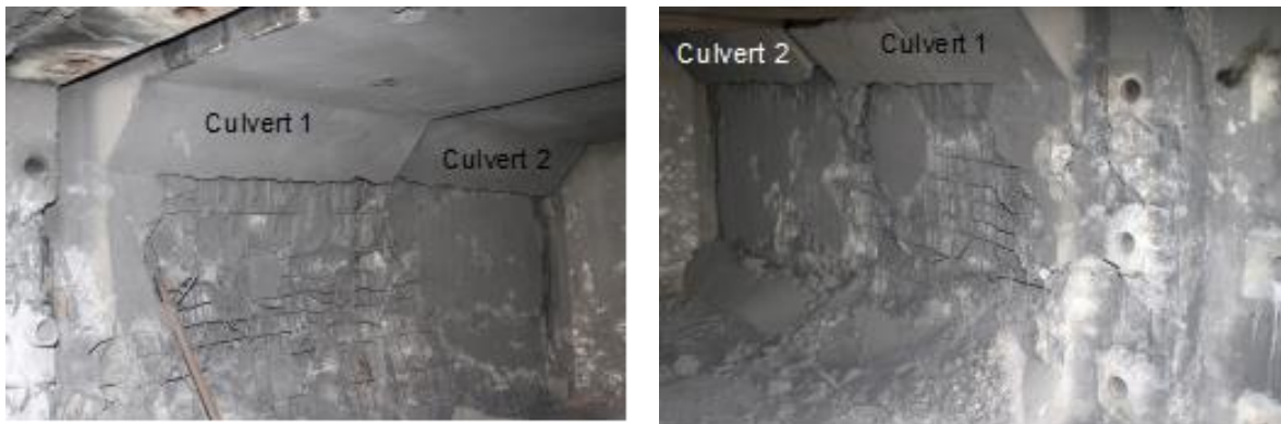
Figure 9. Test results show the significantly damaged east and west culverts
