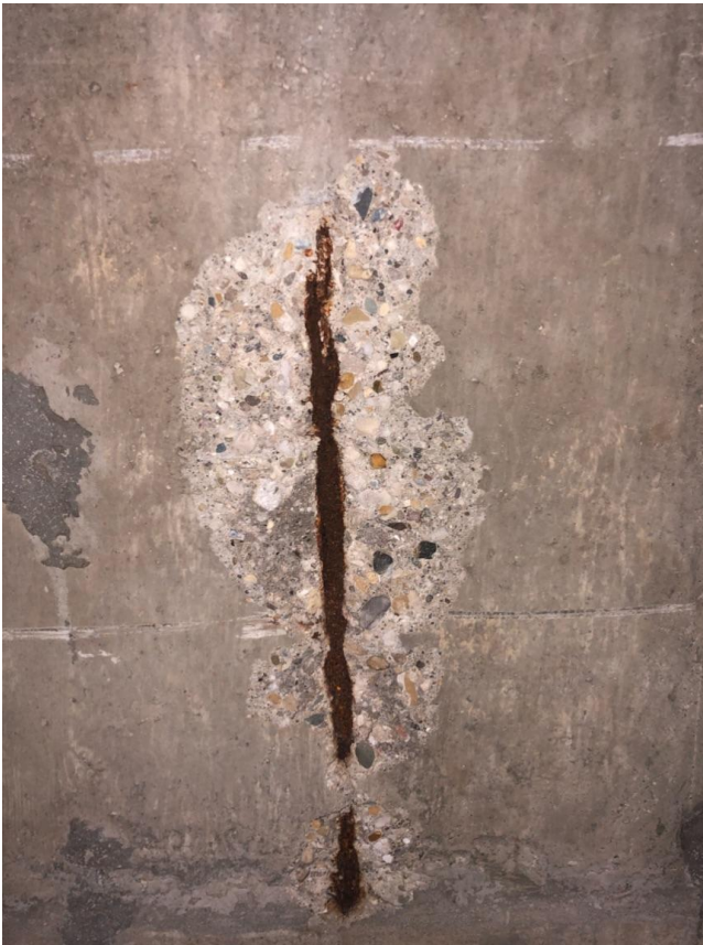
Spalling: Exposed Rebar in Sidewall
