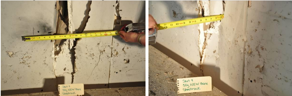
Figure 2-5 – Test 9 (50 g total NEW) Interior Wall Damage at 12” Stand-off
