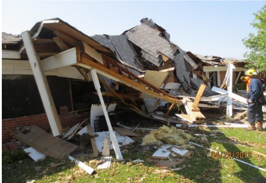
Figure 6. Damage to Eastern Entry of Rest Haven Nursing Home– 650 ft. (K22)
