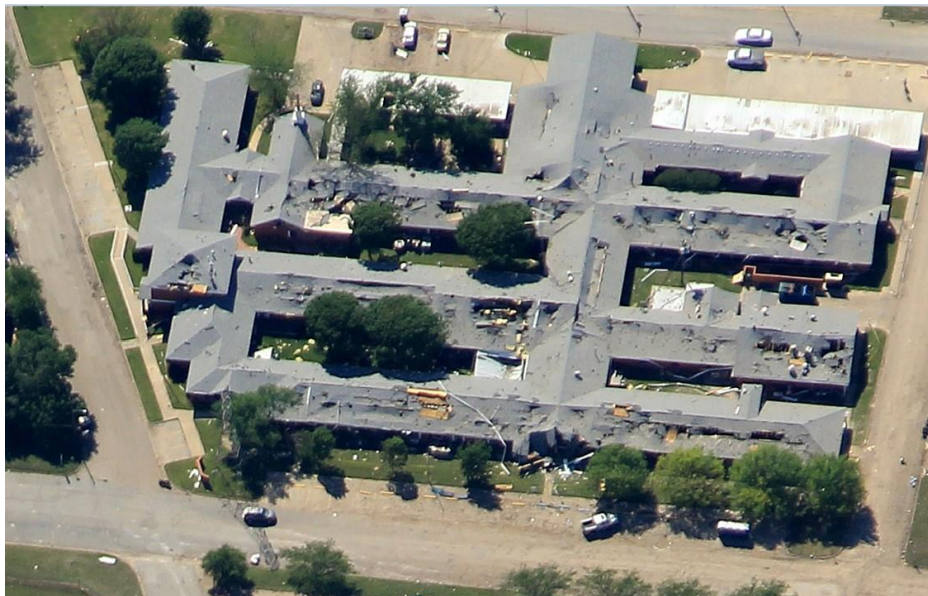
Figure 7. Post Incident Aerial View of Rest Haven Nursing Home (Roof Debris Impacts)
