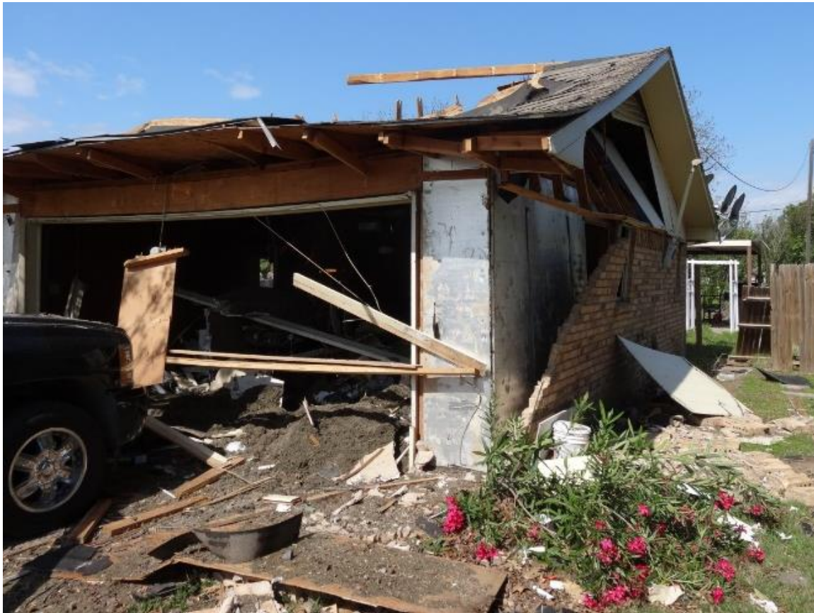
Figure 16. Examples of Observed Residential Damage - 700 ft. (K24)
