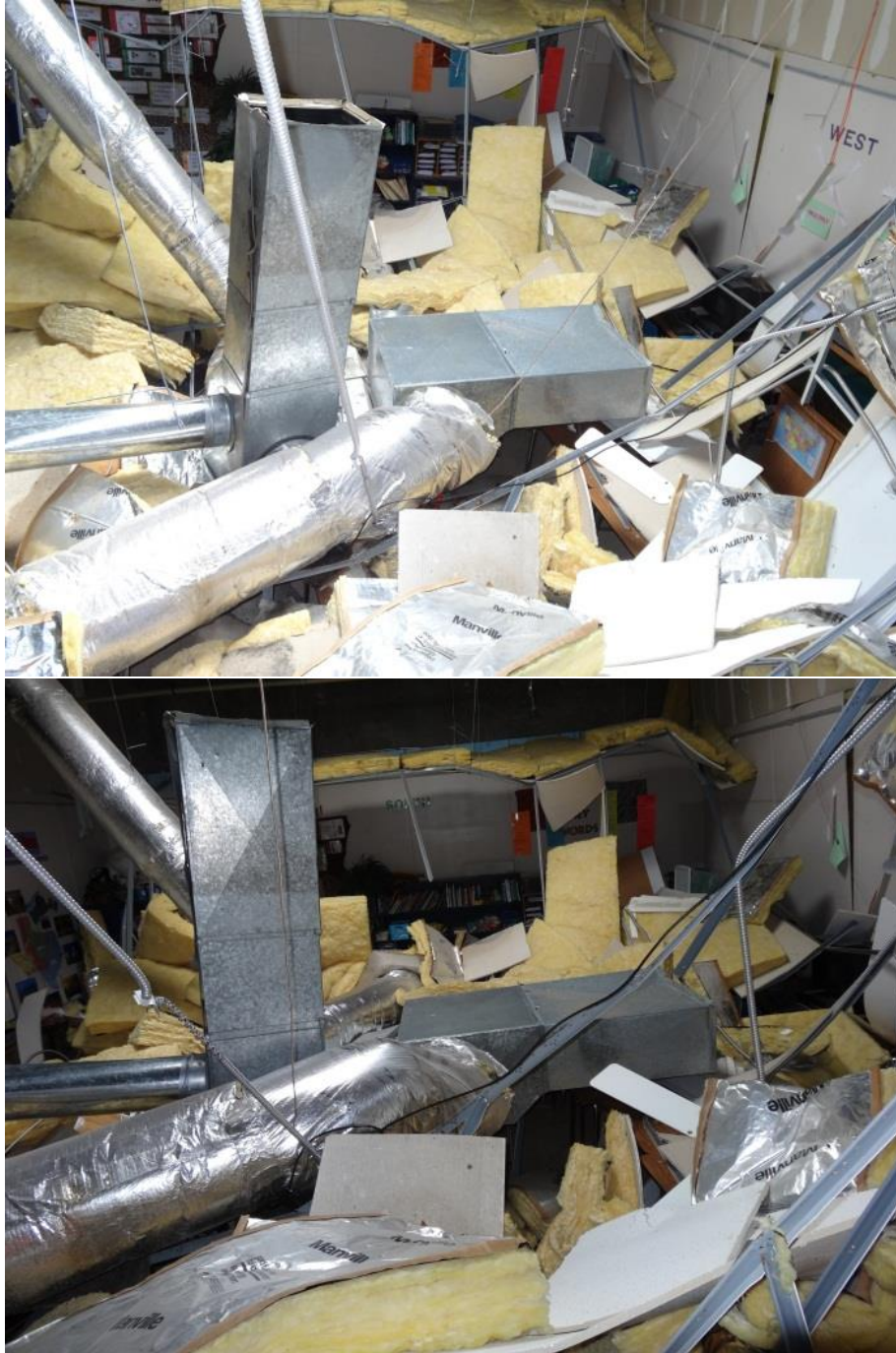
Figure 11. West Intermediate School – Classroom Nonstructural Debris
