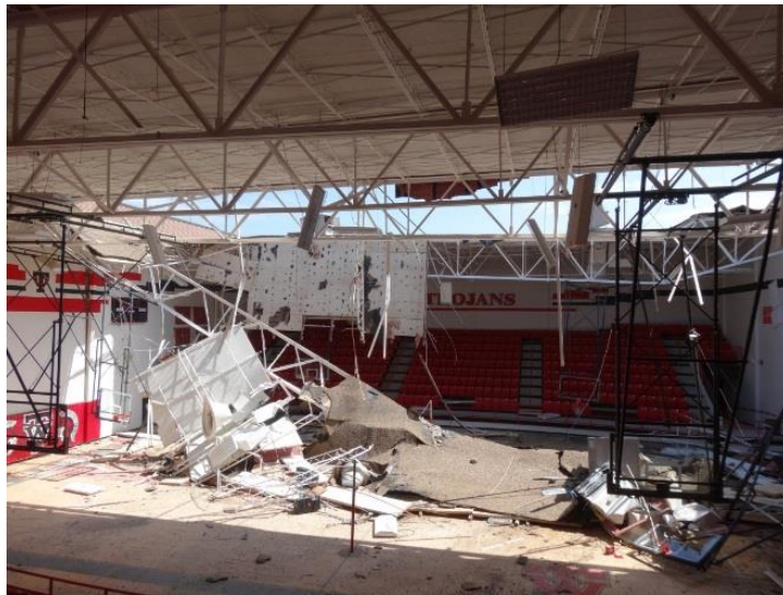
Figure 13. West High School Gymnasium 1 Roof Collapse from South Bleachers
