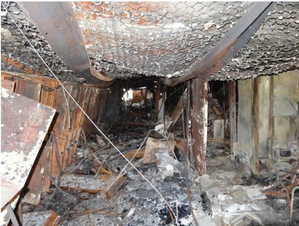
Figure 10. West Intermediate School Interior of Northeast Section that Burned
