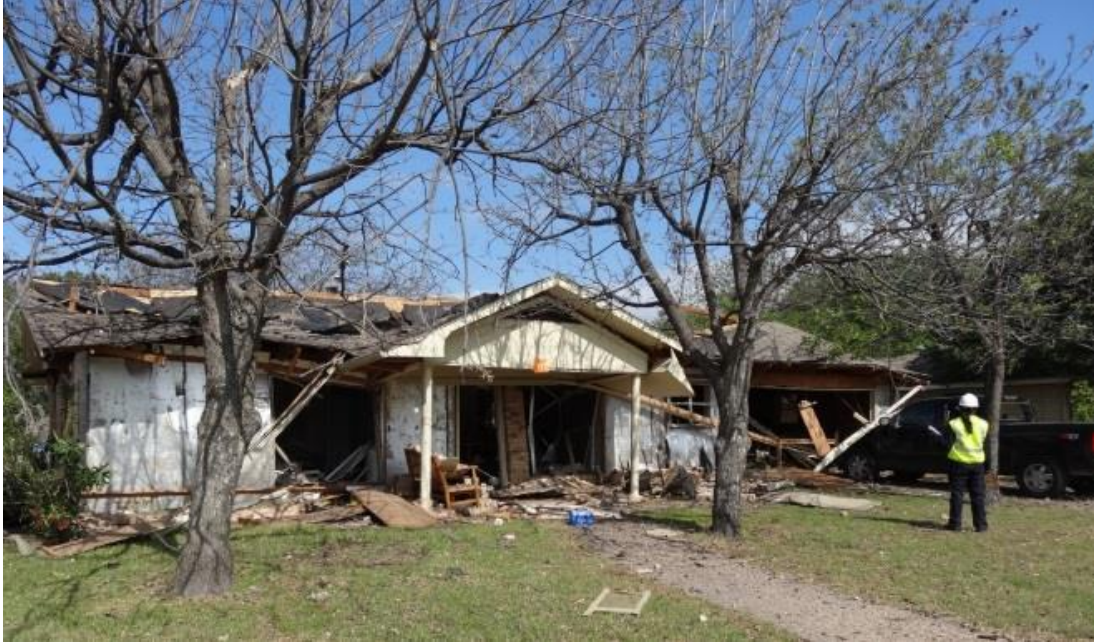
Figure 15. Heavily Damaged Residence - - 700 ft. (K24)
