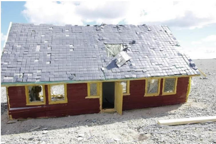
Figure 6 Front wall and back wall of Lykkebo in scale 1:5 after detonation of 350 kg Texit 40 35 m from the house 15
